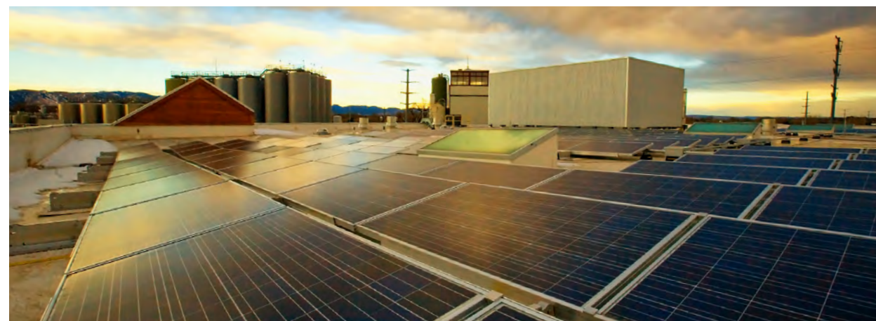
At New Belgium Brewery in Fort Collins, a rooftop solar PV array—the largest privately owned array in the state when it was commissioned in 2010—generates 264,000 kWh of electricity each year.
