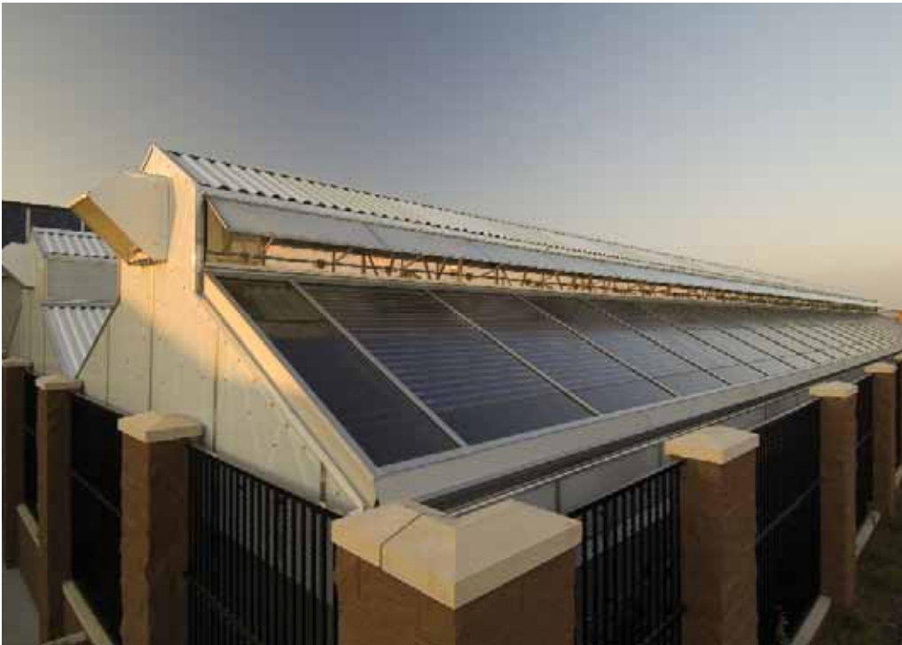
Above and above left: PVs and a bioswale at the McKinney store.
