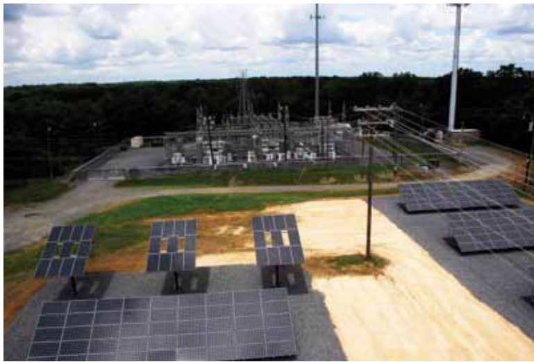
Top: Duke is currently evaluating building new nuclear facilities, similar to its McGuire station shown here, to help reduce the company's carbon emissions.
