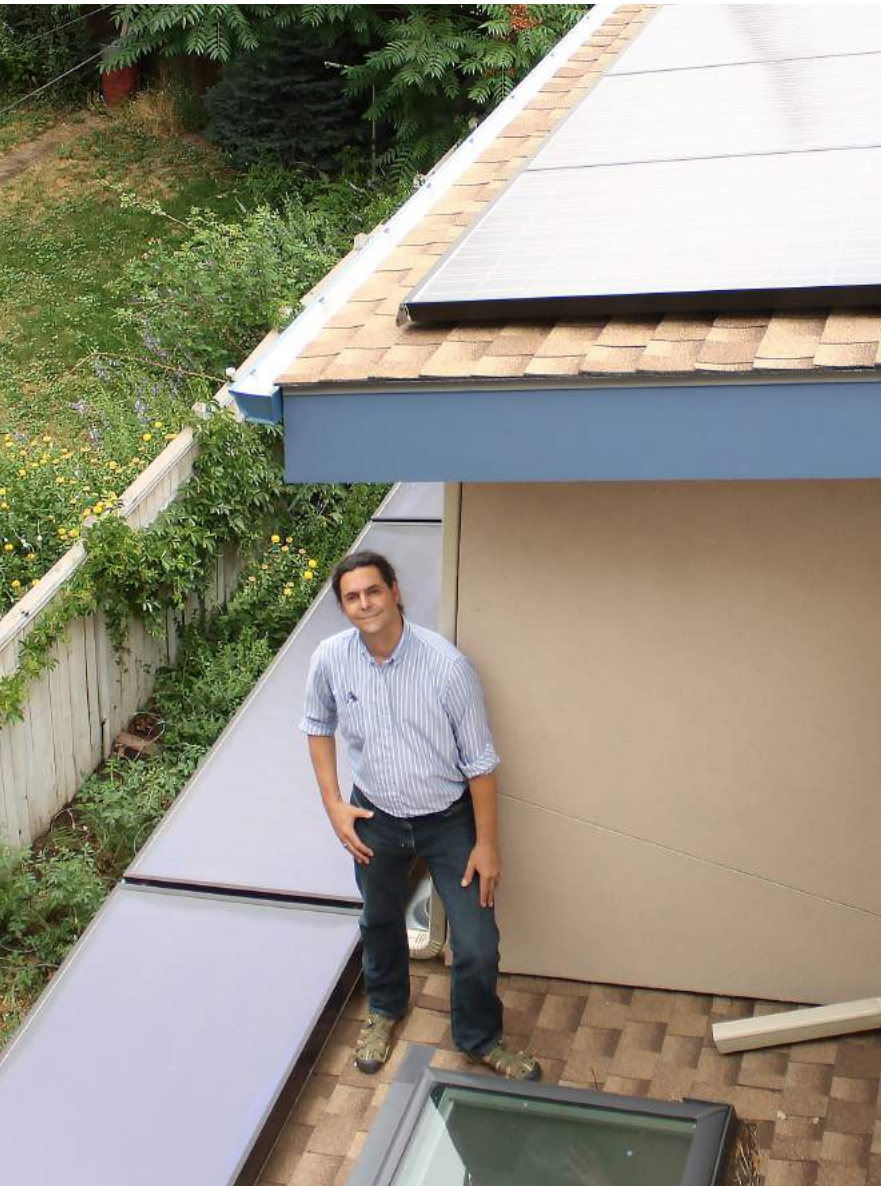
Solar thermal collectors on the lower roof and a solar PV array on the higher roof supply the home's hot water and electricity.
